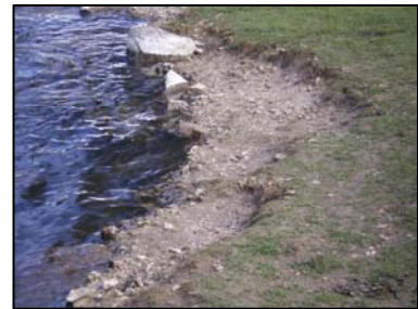
Erosion before project
