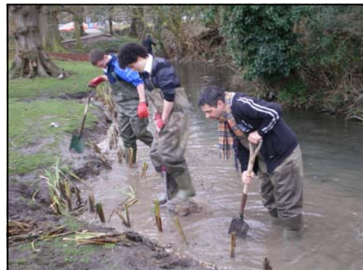
Photos: Top left back stream before project showing inlet sluice. Top right back stream with new log revetments in place (photo in high flow conditions so logs submerged). Above: St. John's School plant backfill behind new log revetments, Left: June 2009 showing backfill plants growing well.
