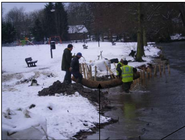
Above: working in January snow to create new sinuous bank profile constructed with coir roll
